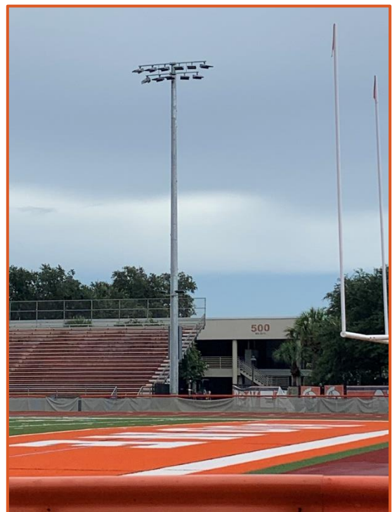
AFTER: New LED Athletic Field Lighting at Boone High School
